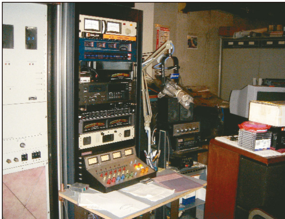
The transmitter room at the archival house.
